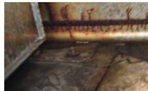
Rust to interior of combi oven before using Citrajets.
